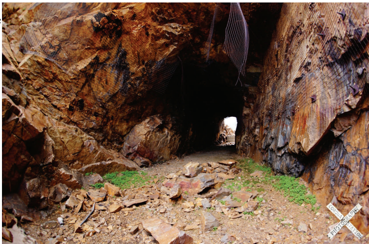
RPRA thanks Travis and Kate Wright's, husband/wife photography team for their most recent photo of the inside of The Needles Eye Tunnel. At CoronaStation.com Photography , we believe in the pursuit of happiness: capturing the grandeur of Rollins Pass while sharing the splendor of the inexpressible.
