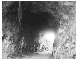
Needle's Eye Tunnel, Wire Mesh is doing its job!
